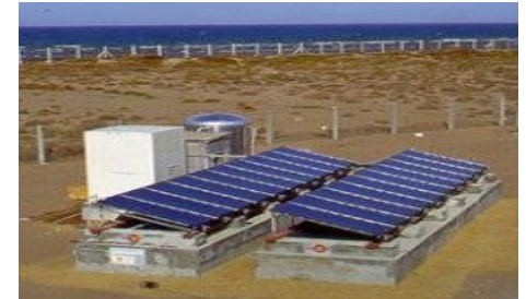
Source: Mage Water Management Desalination installation in Al-Hail in Oman www.bsria.com
