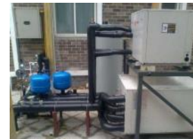
Ground source heat pump
