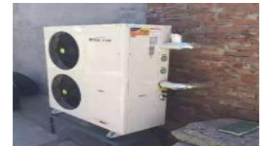
Air Source Heat Pump (ASHP)
