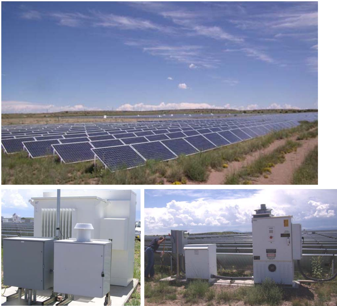
Figure 8. (Top) A portion of a 6.4-MW utility-scale solar field with panels arranged in rows. (Lower right) From right to left: One of the field’s 48 Inverters with attached dc disconnect connected to an intermediate step-up transformer and ac disconnect/meter. (Lower right) One of 12 large step-up transformers for transmission to the grid. Cabinets in foreground house instrumentation.
