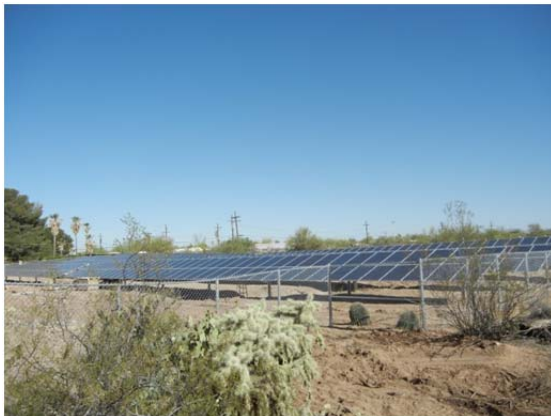
Figure 9. A 140-kW commercial-scale PV farm under construction. It will supply power to a water-utility office and garage. Installations of this type are one example of distributed generation.
