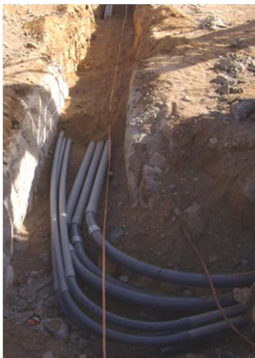
Figure 4. Copper-concentric-neutral power cables and bare-copper grounding conductors connect turbine towers.
