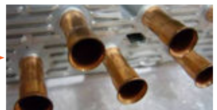
Air Conditioning Tubes
